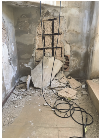
Figure 14. Corrosion effects detected on the bell chamber at a quote of 40 m from the ground level.
