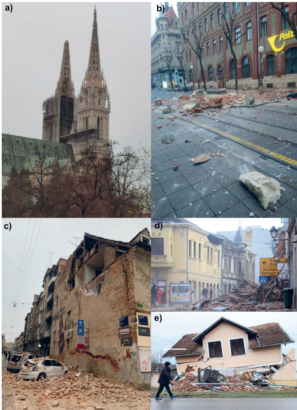
Figure 2. Some examples of earthquake damage from 2020 (Croatia): a Zagreb cathedral – broken tower top; b Zagreb main post office; c Zagreb old town; d Petrinja city – main street area; e Petrinja city wider area – collapsed family house.
